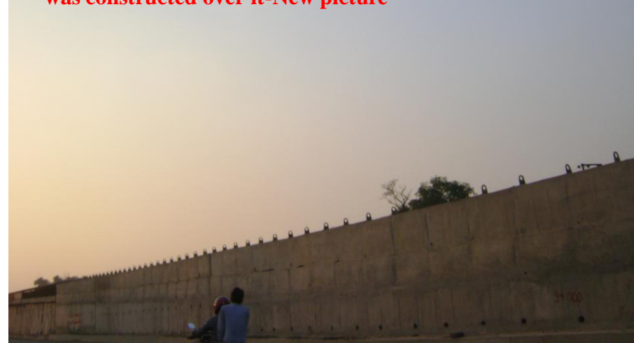
The old dumping site in brick kiln at Ummari village was made empty and Illegally dumped in the slop of Over-bridge at Matiyari Chauraha, Lucknow and road was constructed over it-New picture
